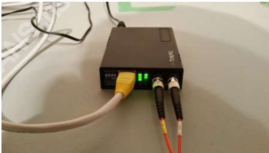
Figure 10 - Fiber Optic Link Setup Using Media Convertors.
