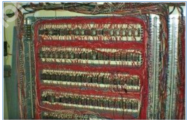
Figure 7 Picture of Factory Relay Rack ( http://www.blog.beldensolutions.com/wp-content/uploads/Old-Relay-System-300x195.jpg )
