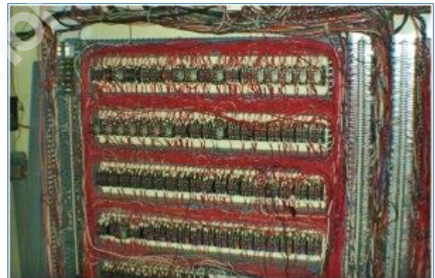
Figure 7 Picture of Factory Relay Rack ( http://www.blog.beldensolutions.com/wp-content/uploads/Old-Relay-System-300x195.jpg )
