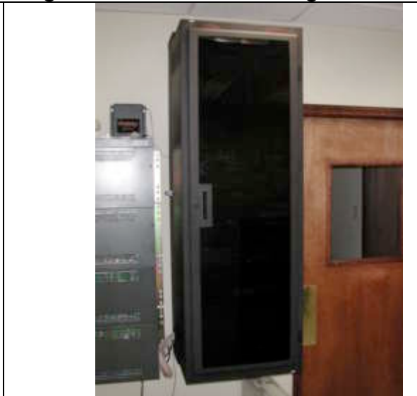
Figure 3.4 Cabinet housing firewall
